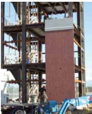
Precast concrete panels were used to enclose the Barnstable airport control tower.
